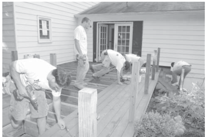
Sears and Kmart volunteers install decking outside Ryan’s room with Gilday Construction providing technical oversight.
